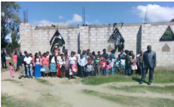
Pastor Geoffrey and his congregation in front of their church that needs a new roof.
